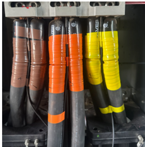
Figure 11 - Sensors attached directly to 600VAC busbar with rubber tape
