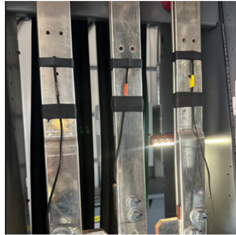
Figure 10 - Sensors attached directly to insulated cables
